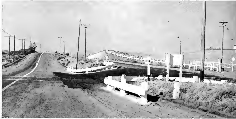
Guard rail fabricated at factory for curve and difference in elevation of two roadways
